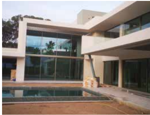
SINGLE-FAMILY HOUSE VALE DE LOBO Loulé, Portugal Architect Agency: João Cabrita - Arquitecto Fabricator: Lusocaixilho
